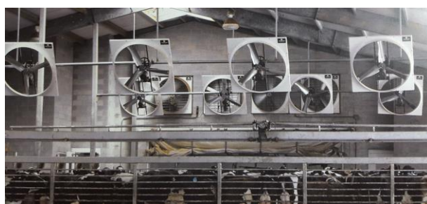
FIG. 9. Circulation fans and sprinklers over holding area.
